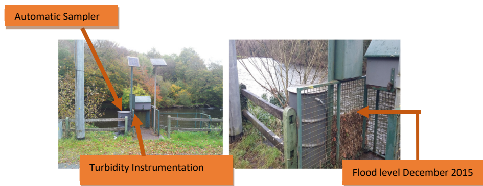
Figure 6: River Monitoring Installation at Curranure Gauging Station, River Bandon
